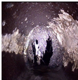
Grease build up
