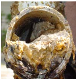
Grease build up
